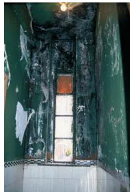
Fig 3: Peeling paint in degraded housing stock
