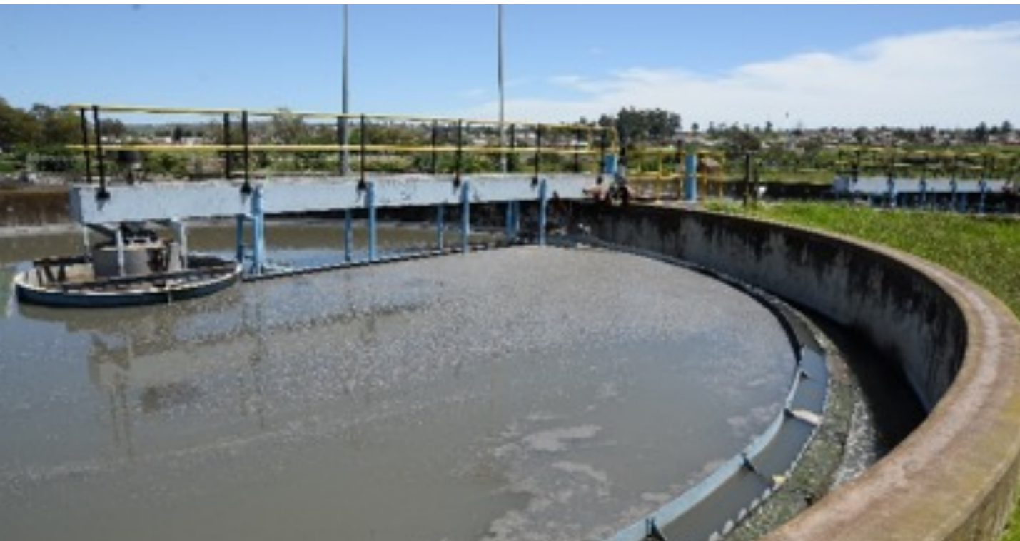
Wastewater Treatment Plant
